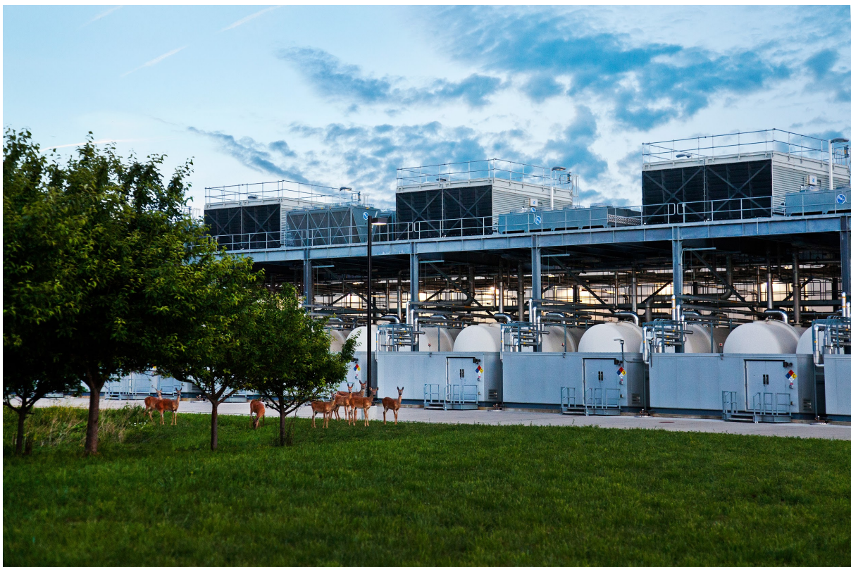
Figure 2. Photograph of the Council Bluffs data centre, with a family of deer in the foreground.
